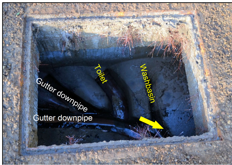
Typical Combined Sewer in Peasmarsh
