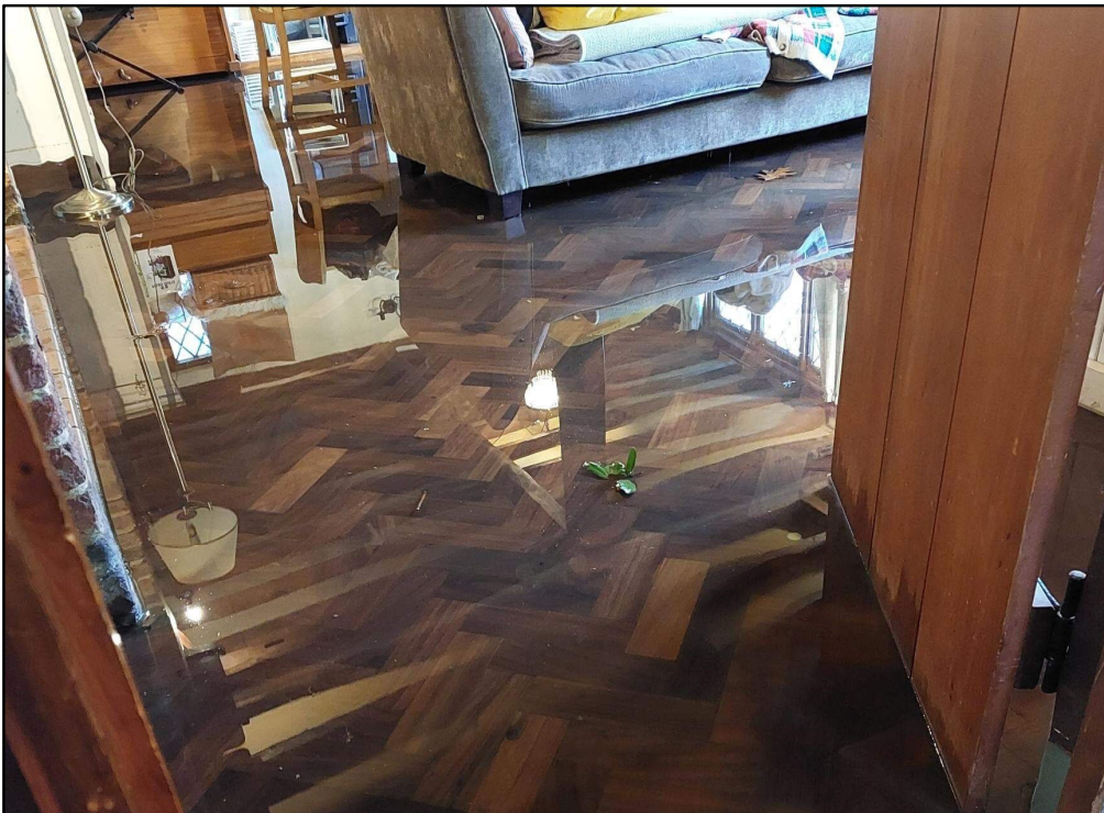
Internal Flooding of a House on the A268 near Mill Lane following rain event
